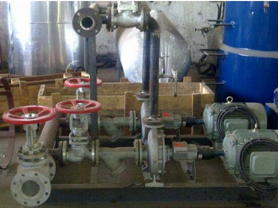
2 Nos. Circulating Pump Assy.
