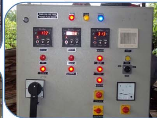
Control Panel For Automatic Operation
